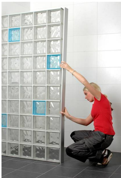
Glue the metal end channel to the side and top of wall.
